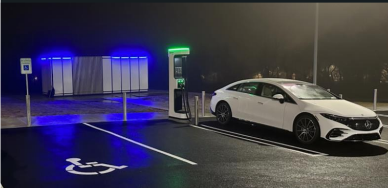
Upgraded on-site demo installed
